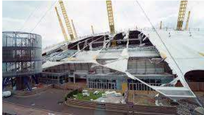
Figure 3: A photo of the damage to London’s Millennium Dome following Storm Eunice on the 18 th of February 2022.
